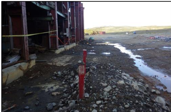
Figure 18.–Piezometers installed near mill building to monitor groundwater.
